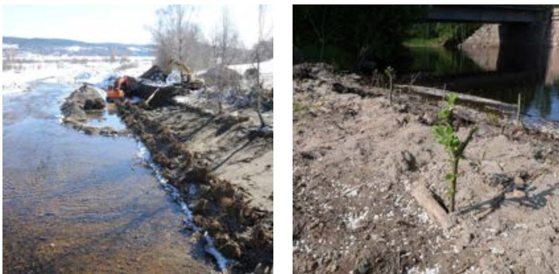
Figure 25. Implementation of the large wood structure in Gjødingelva (Hurdal) during the spring of 2023. To the left: excavation work, 31.3.23. To the right: planting of tree seedlings, 2.6.23. Photos: Helge B. Pedersen (Huvo).
