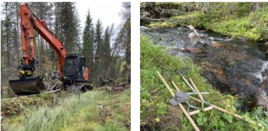
Figure 18. a) Excavations in the field for peatland restoration and b) use of the manual Hartijoki method in the stream restoration. This kind of restoration work starts with a hoe, a scraper to open up the impacted bottom and continue with adding and/or rearranging gravel in the streams (Photos: Antti Karppinen / Metsähallitus' Wildlife Service of Finland).
